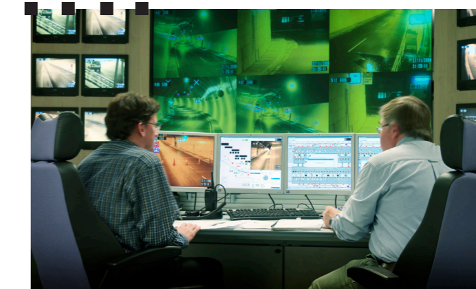
Dublin Port Tunnel control centre
