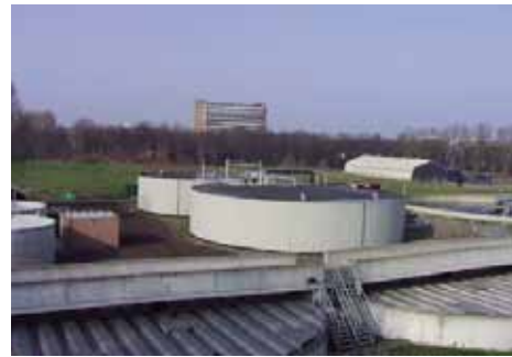
Figure 4 Nitrification reactor (foreground), denitrification reactor (background)
