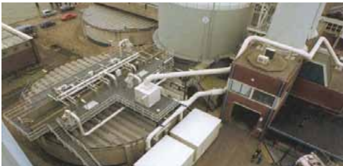
Figure 12 Reactor left, methane storage background
